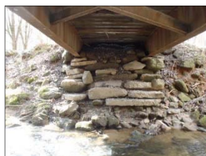
Typical LOCBR project substandard super and substructure
